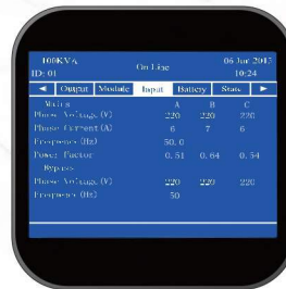
UPS Cabinet Control Panel
